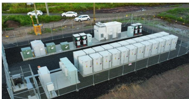
The high voltage battery installation will have rows of modern, modular battery banks like this one, with additional communications and electrical switching equipment.
