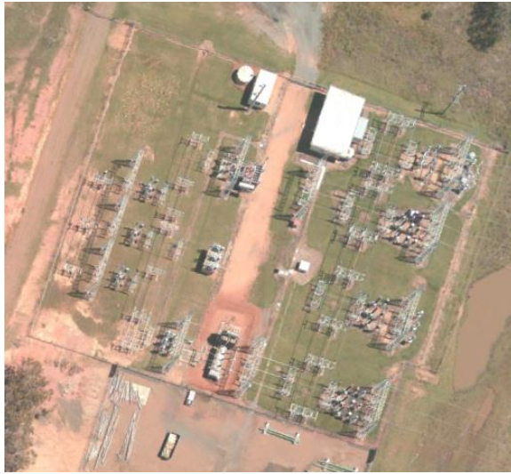
Figure 1: ROAMES image of Kilkivan Substation
