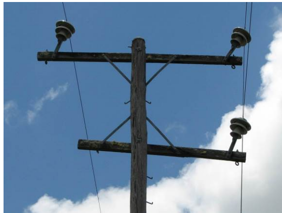
Figure 12 - 66kV delta pin construction
