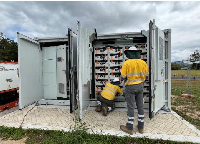
Fig 3 – Inspecting and testing the microgrid batteries.
