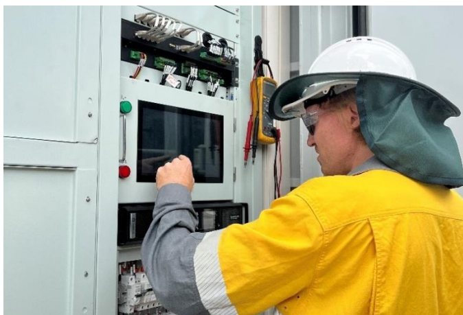
Fig 1 – Jake runs through operating procedures on the microgrid during commissioning.
