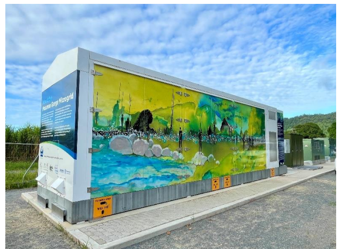
Fig 2 - The Mossman Gorge Microgrid's BESS unit has been transformed with the application of the wraps.
