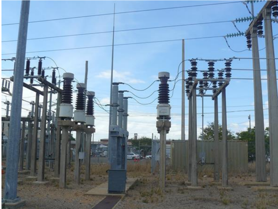
Figure 18 Photo showing the aerial bus spanning the bus tie circuit breaker
