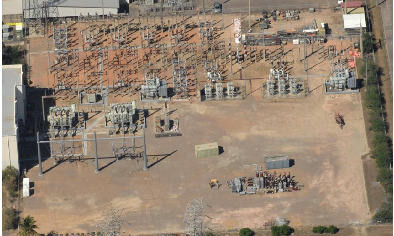
Figure 16 Aerial image of Garbutt Substation
