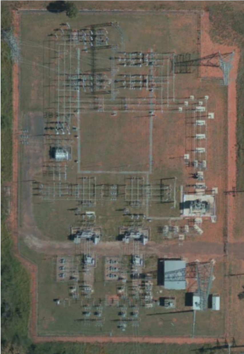
Figure 3: Chinchilla Substation (geographic view)
