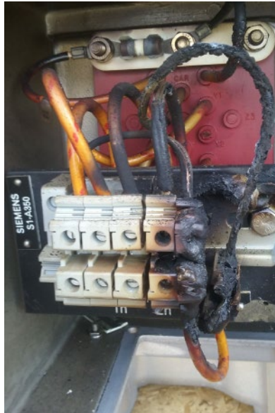
A1 terminal inadvertently left disconnected
