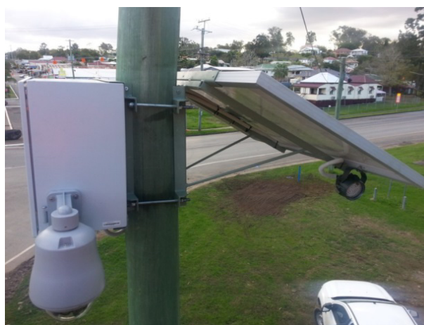
Figure 12: Representative Example - Unacceptable Security Camera Installation
