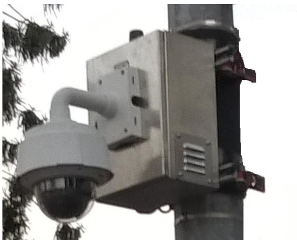
Figure 9: Representative Examples - Temporary - Rapid Response Security Camera Installation
