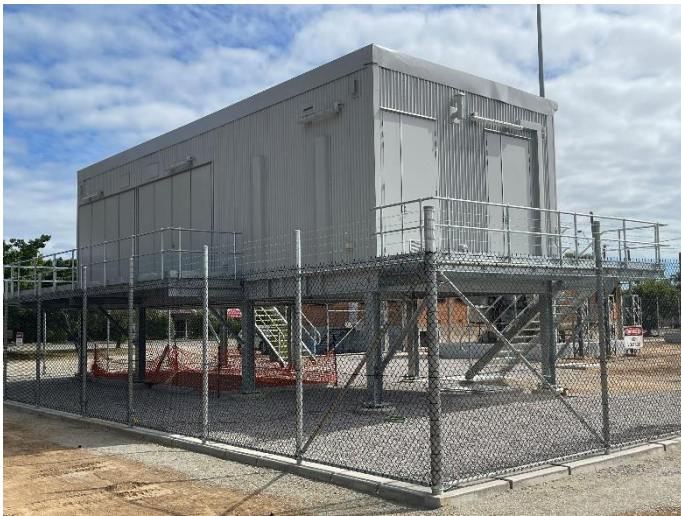
Fig 3 – The new modular switching building at Cranbrook substation.
