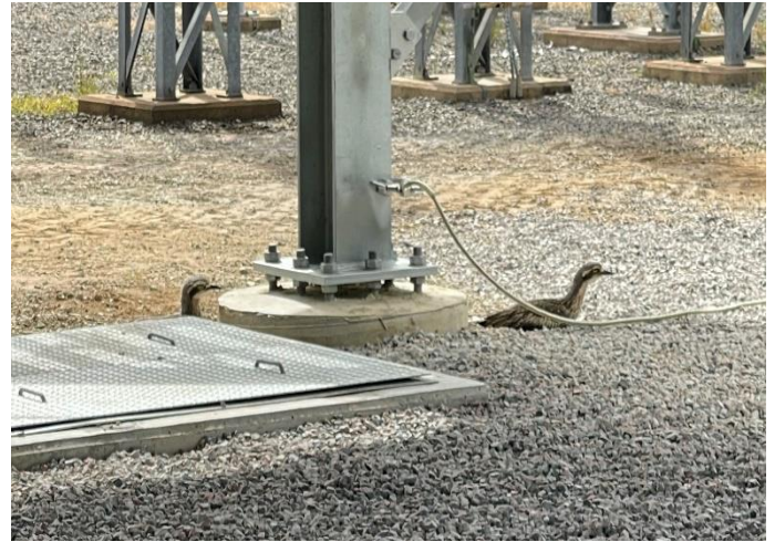
Fig 4 – The resident family of curlews have moved back into Cranbrook substation yard.
