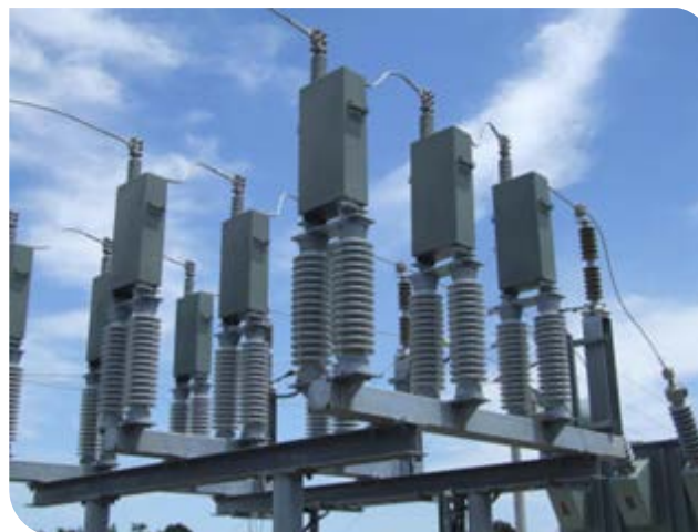
Outdoor AFLC equipment in an Ergon Energy substation
