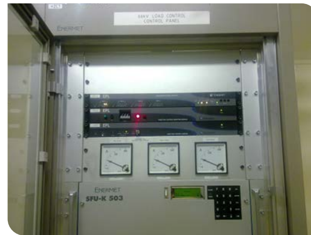
Transmitter and controller panel for AFLC.
