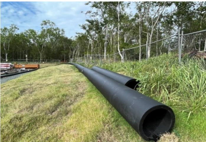
Fig 5 - The new Whitsunday Regional Council sewerage pipe will be installed when weather permits.
