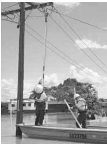
Crews across southern and central Queensland undertook plenty of preventative switching during the past summer’s long-running flood crisis. Here a crew is disconnecting by boat in Rockhampton.
