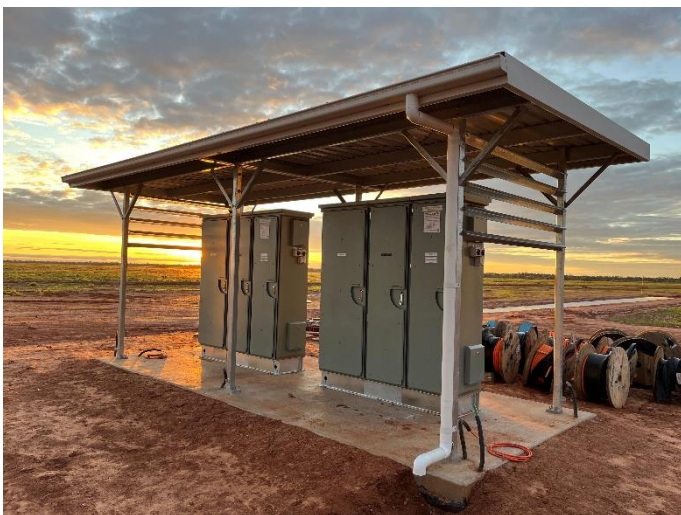
Fig 4 – Cabinets housing the distribution boards that will connect the solar farm into the network.
