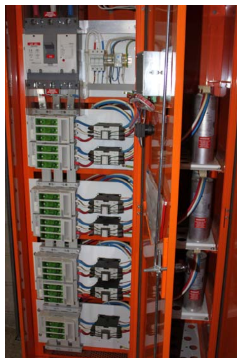
Power-factor correction equipment in the older part of the shopping centre.
