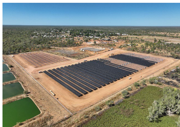
Aerial view of racks and panels
