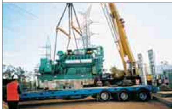
Construction started on a new $12 million power plant in Moranbah, providing a boost for regional Queensland economies, and leading the way with the use of coal-seam gas as an environmentally friendly fuel source.
